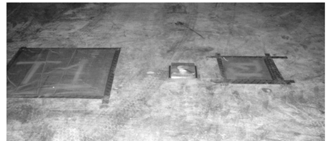
Fig. 3.2—Even though plastic sheet tests can show no evidence of moisture, calcium chloride tests conducted on adjacent concrete can indicate moisture vapor emission rates as high as 13 lb/1000 ft 2 /24 h (6.3 kg/100 m 2 /24 h) (Suprenant 2003b; Kanare 2005).
