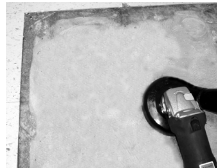
Fig. 3.7—Surface preparation using grinder before installing a moisture vapor emission test. (Courtesy of Peter Craig.)
