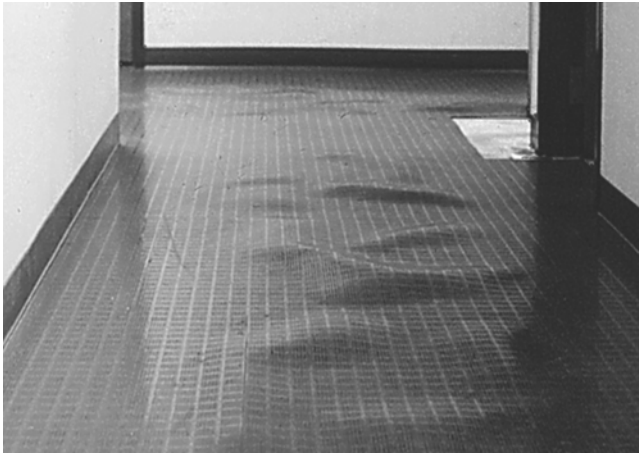
Fig. 1.1—Debanded sheet flooring due to moisture in the concrete slab. (Courtesy of Peter Craig and Herman Protze III.)
