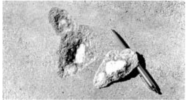
Fig. 11.7—A popout is a small fragment of concrete broken away from the surface of a slab due to internal pressure, leaving a shallow, typically conical, depression (PCA 0113).
