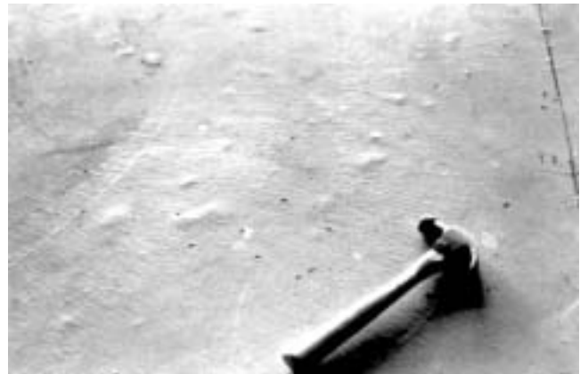
Fig. 11.8—Blisters (courtesy of NRMCA).
