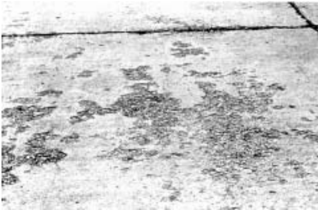
Fig. 11.5—Scaling is the loss of surface mortar, usually exposing the coarse aggregate (PCA A5273).
