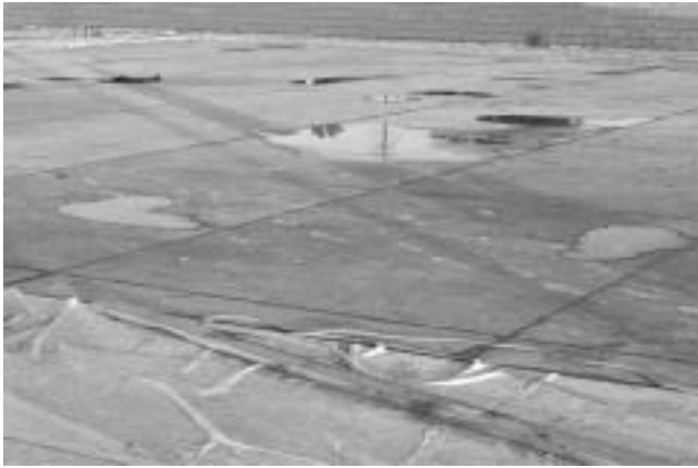
Fig. 11.11—Low spots in a slab after rain shower (courtesy of Eldon Tipping).
