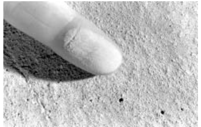
Fig. 11.4—Dusting is evident when a fine, powdery material can be easily rubbed off the surface of a slab (PCA 1297).
