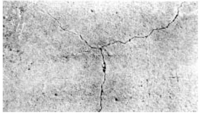
Fig. 11.1—Drying-shrinkage cracks such as these are a frequent cause of complaint (PCA A5271).
