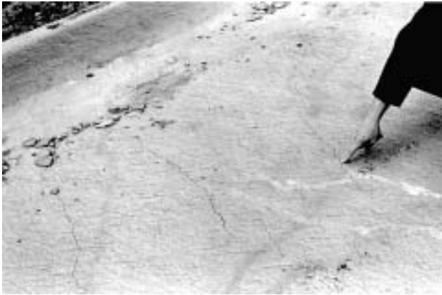
Fig. 11.2—Plastic-shrinkage cracks are caused by rapid loss of mixing water from the surface while the concrete is still plastic (PCA 1311).
