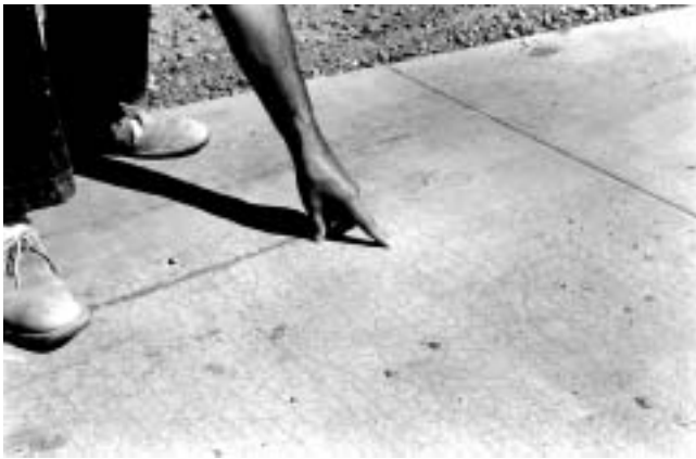
Fig. 11.3—Crazing is a network of very fine superficial surface cracks (PCA 4099).
