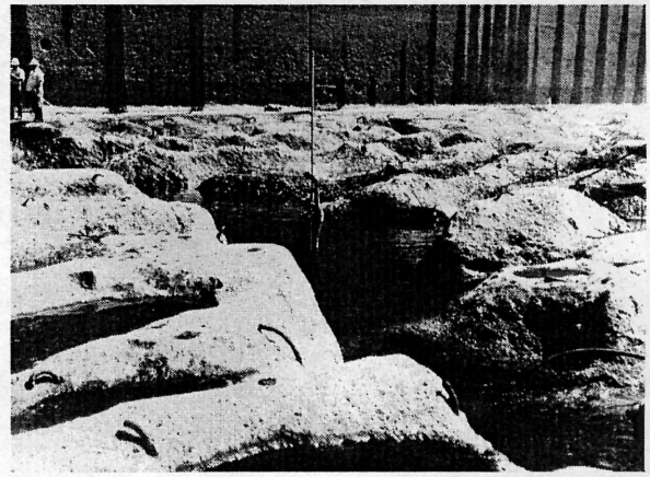
Fig. 3.4-Erosion of stilling basin floor slab, Dworshak Dam
