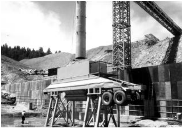
Fig. 5.1—Partial conveyor system to hopper on dam.
