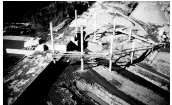
Fig. 5.4—Conveyor delivery of conventional concrete on separate belt parallel to wider RCC belt.
