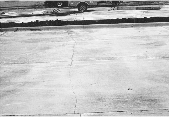
Fig. A.1.8—Shrinkage cracking
