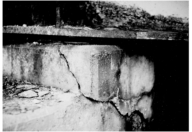
Fig. A.1.4—Diagonal cracks
