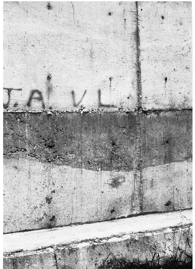
Fig. A.3.6—Close-up scaling (severe)
