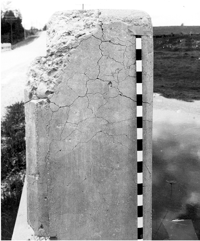
Fig. A.1.6c—Pattern cracking (wide)
