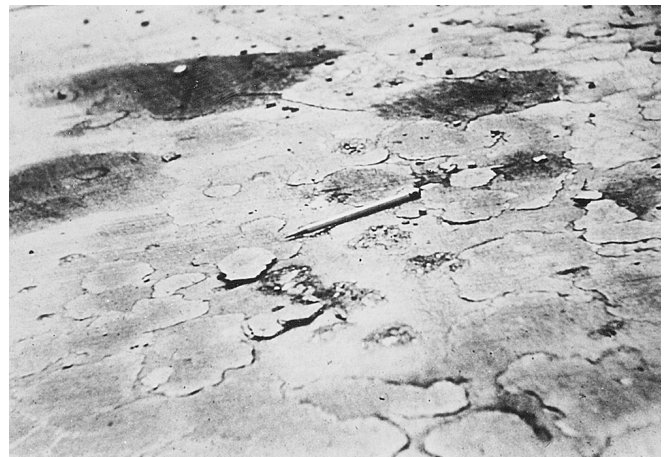
Fig. A.2.2—Shrinkage cracking
