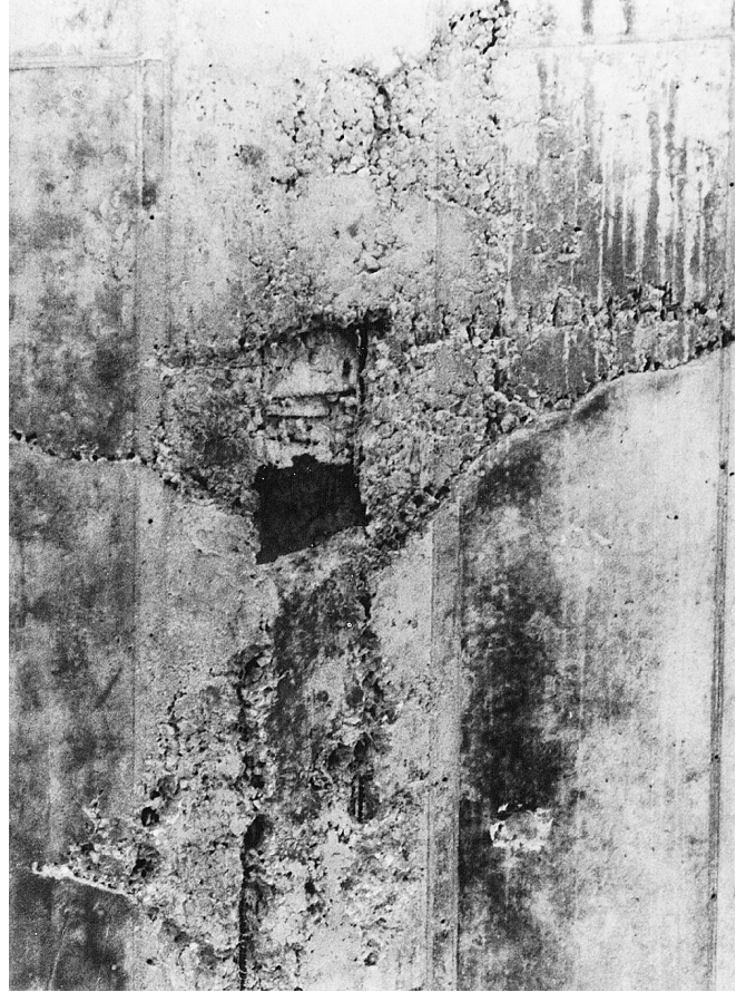
Fig. A.3.5—Cold joint
