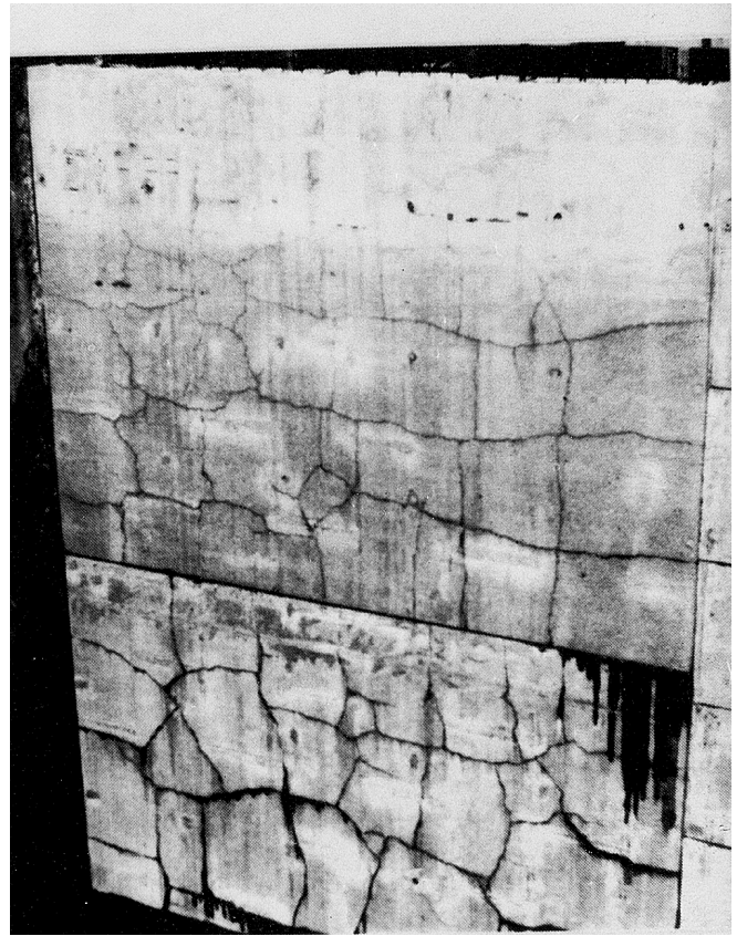
Fig. A.1.6e—Pattern cracking (restraint of volume change)
