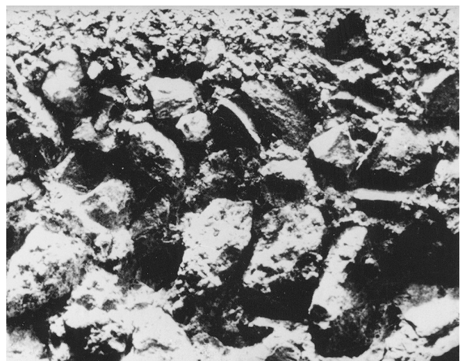
Fig. A.2.3—Cavitation damage
