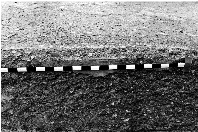
Fig. A.2.20.3b—Close-up scaling (severe)
