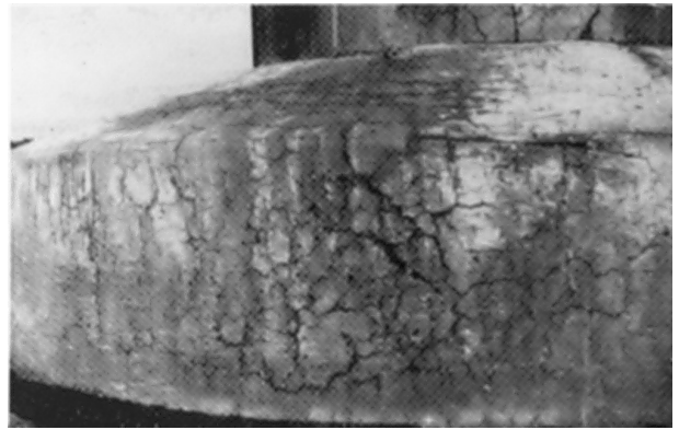
Fig. A.1.6f—Pattern cracking (alkali-carbonate reaction)
