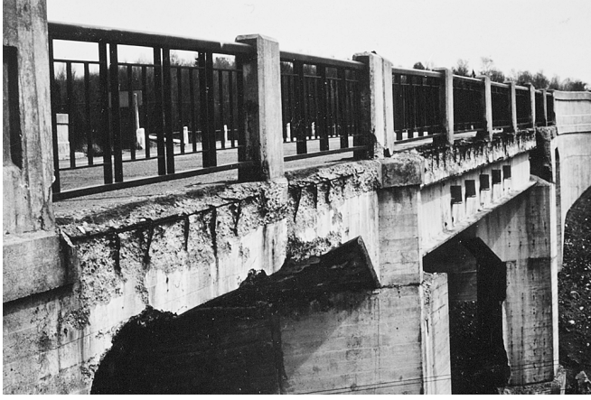
Fig. A.2.5—Corrosion damage
