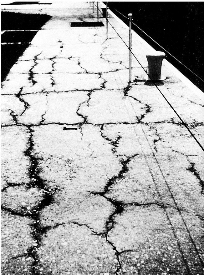
Fig. A.1.6d—Pattern cracking (alkali-silica reaction)
