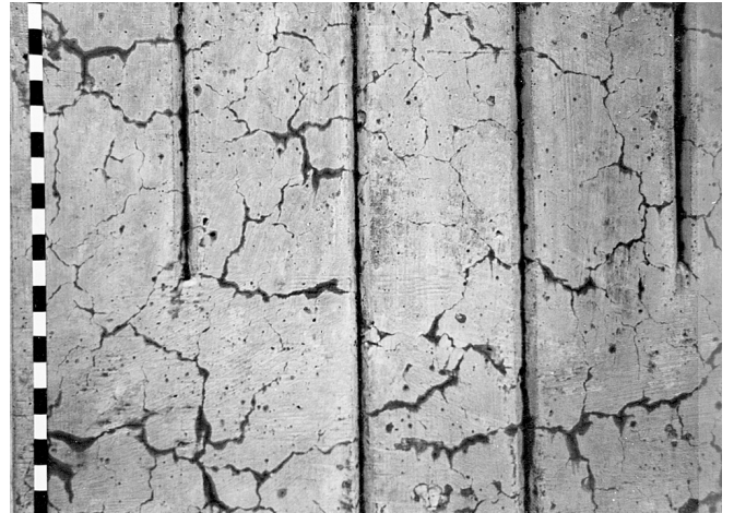
Fig. A.1.6a—Pattern cracking (fine)
