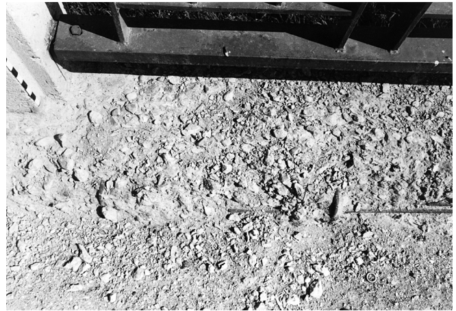
Fig. A.2.20.4b—Close-up scaling (very severe)
