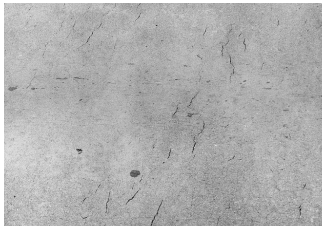
Fig. A.1.7—Plastic cracking
