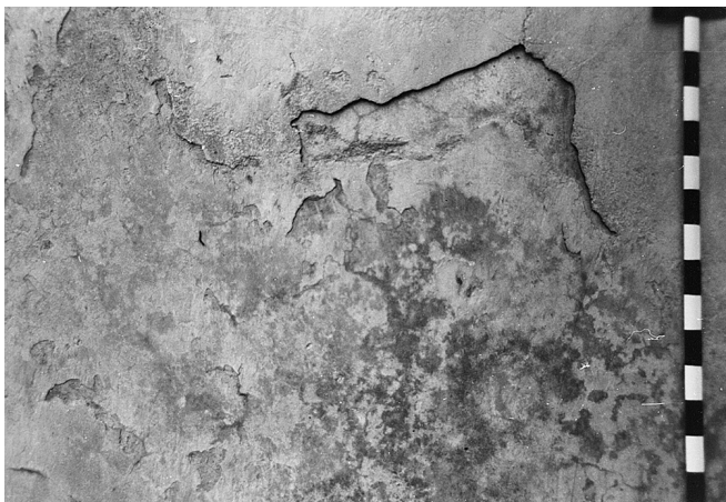
Fig. A.2.18b—Peeling (close up)
