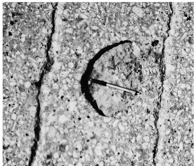
Fig. A.2.21.1—Small spall
